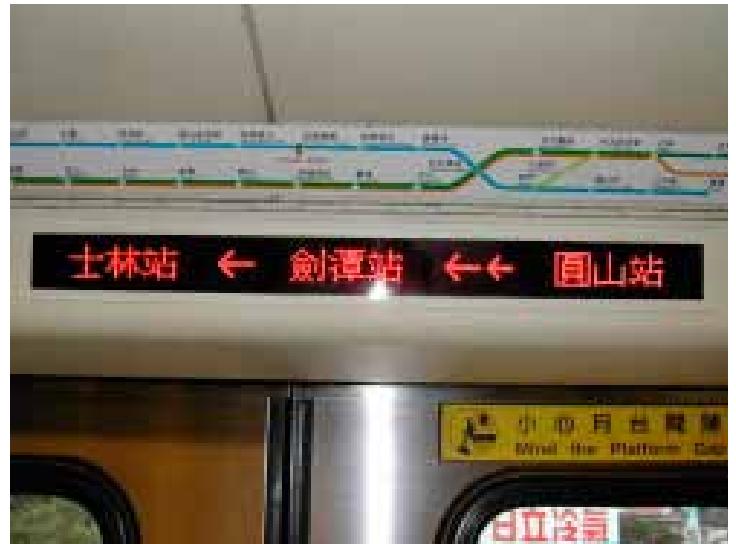
Passenger Information Systems - bi-lingual public address system, bi-lingual visual destination, station and train route indicators.
